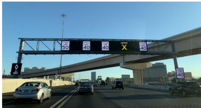
Image: a “first of its kind in Nevada” active traffic management (ATM) system on I-15 through downtown Las Vegas.
