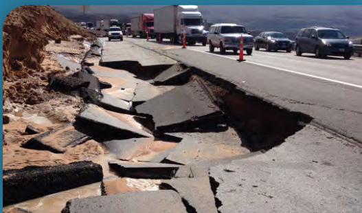
I-15 flood damage, September 2014
