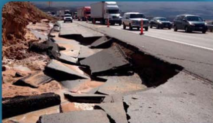
I-15 flood damage, September 2014
